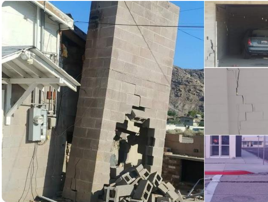
Figure 20. Damage to a masonry house in Trona after the M 7.1 earthquake (Source: Eytan Wallace via Twitter)
