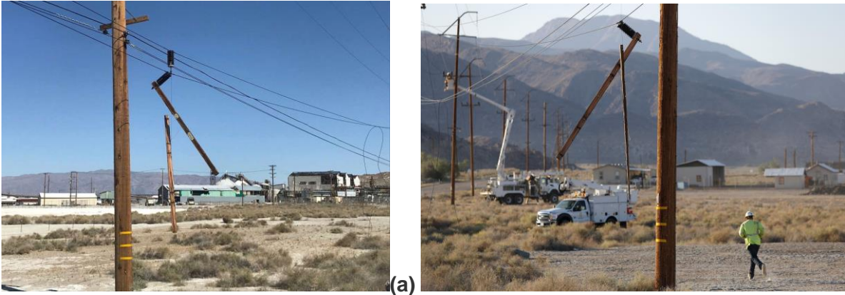
Figure 38. (a) A utility pole in Trona was damaged during the earthquake 32 ; (b) Workers repair damaged utility lines in Trona, CA (AP Photo/Mario Tama | Getty Images 33 )
