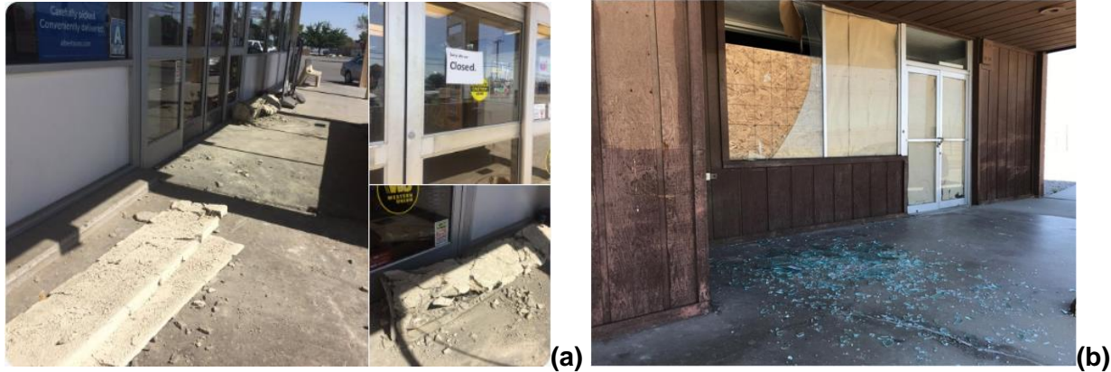
Figure 15. (a) Fallen concrete panels at a building in North Ridgecrest (Source: Karen Hua via Twitter ); (b) Glass facade damage in retail building due to M 6.4 event (Source: AP)
