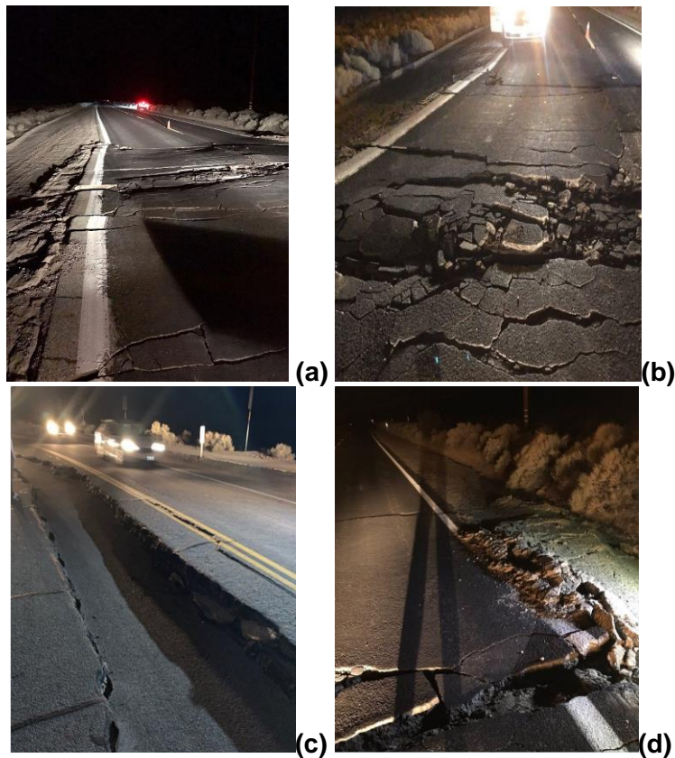
Figure 33. (a) Several cracks on the SR 178 WS between Trona and Ridgecrest after the M 7.1 event. The road was closed for repairs; (b) Details of the cracks 26 ; (c) Other picture of the cracks 27 ; (d) Rockfall cleared on SR 178 between Trona and Ridgecrest but route still closed for temporary repair 28
