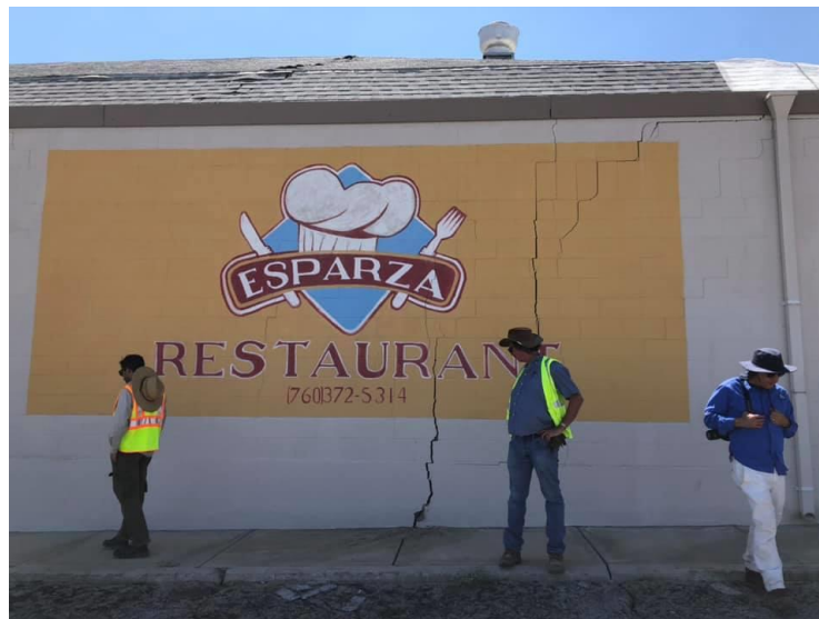
Figure 16. Cracks in masonry walls in Trona following the M 7.1 event (Photo by Christine Goulet, SCEC)
