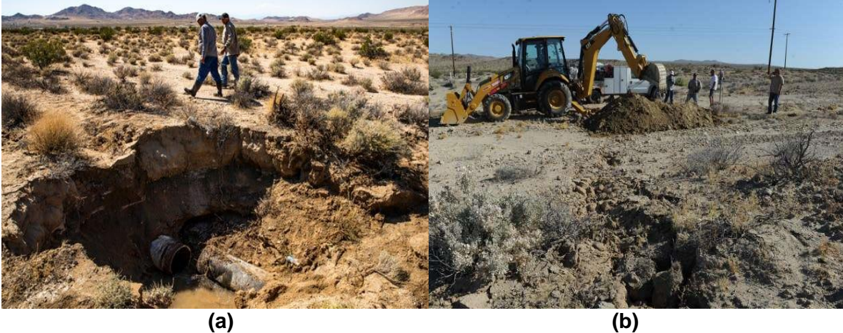
Figure 40. (a) Exploded water pipe reported during the M 6.4 event, consequently forming a crater near Ridgecrest (Source: AP Photo/Etienne Laurent, EPA-EFE 36 ; (b) Crews dealing with a water main that ruptured during the earthquake 37
