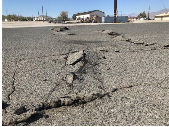
Figure 32. A road in Trona slightly damaged during M 6.4 event (AP Photo/M. Hartman 25 )
