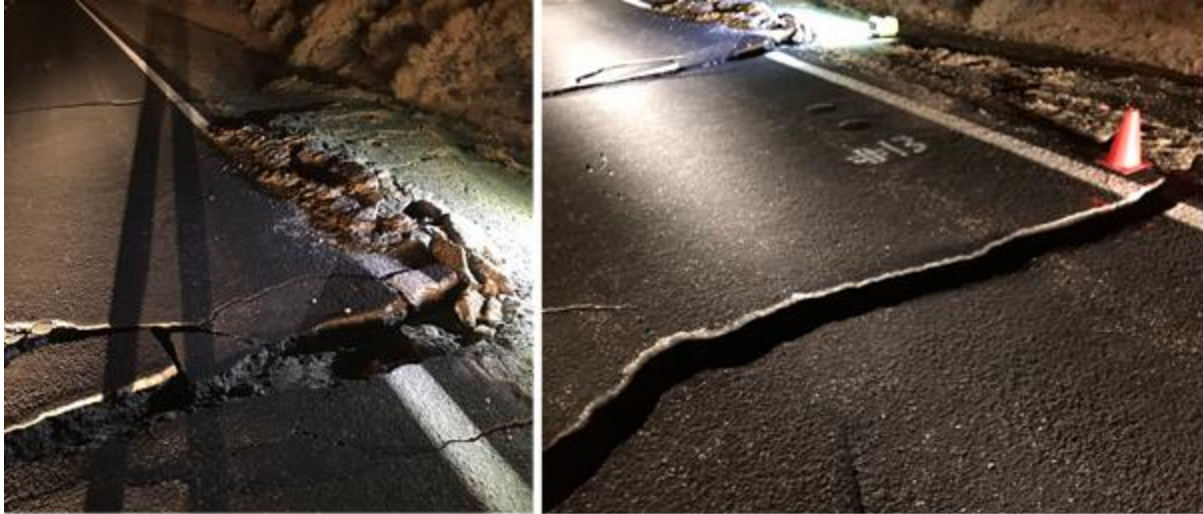
Figure 49. SR 178 near PM (post mile mark) 8.5 Caltrans crews making repairs to patch road before open to traffic 57 (picture taken 12:53am 07/06/2019)
