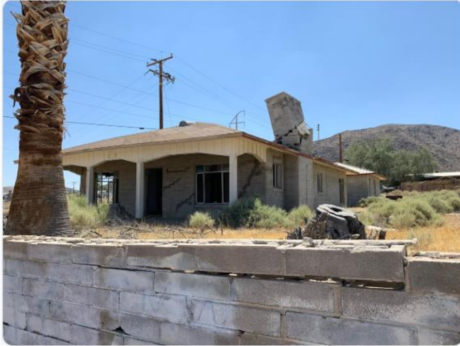
Figure 24. Broken masonry chimney and damaged masonry walls (Source: Ken O'Doll via Twitter)
